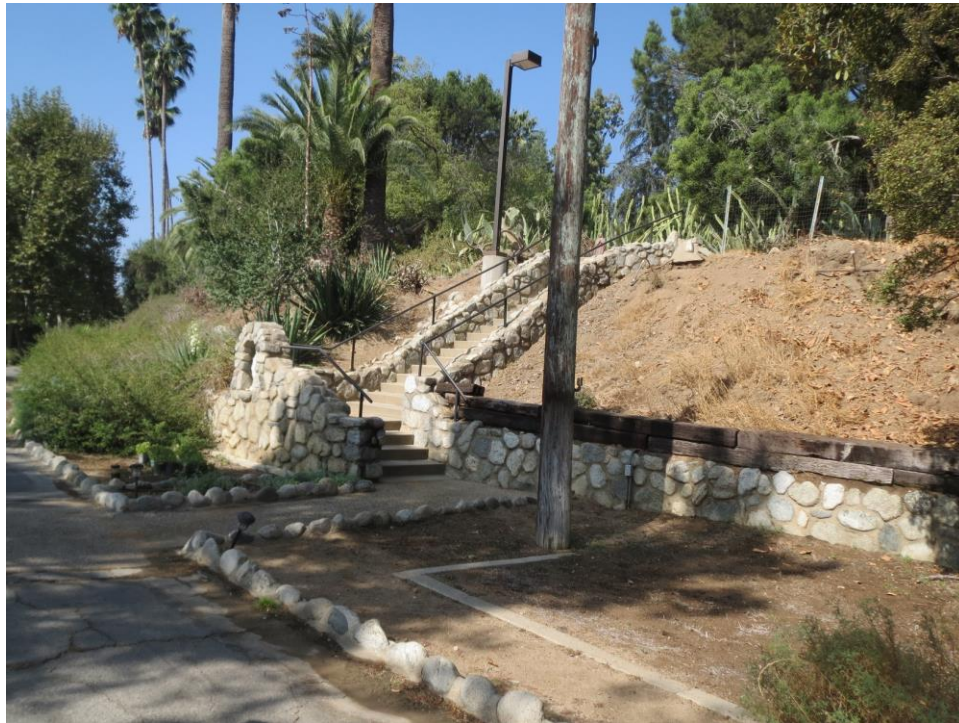
Figure 47. Example of typical stone retaining wall, stair and lined path. View looking northwest (IMG_4667)
