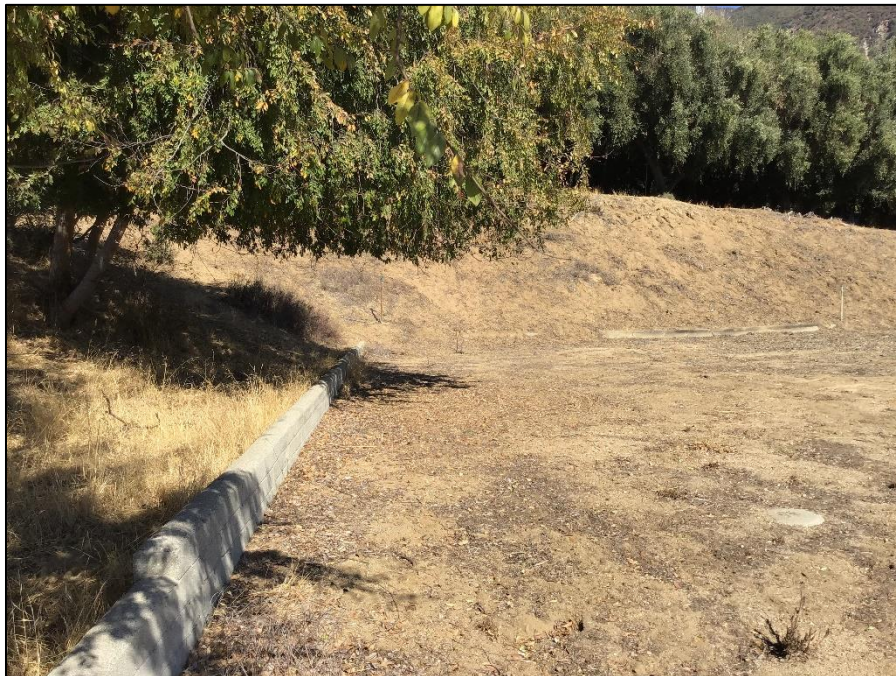
Figure 9. View of retaining walls along northwest corner of proposed Project site; view facing north/northeast.
