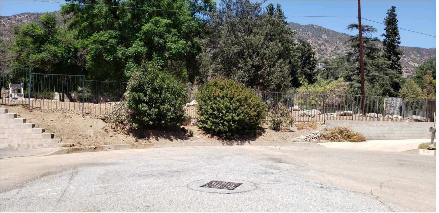
Runoff and Erosion from Water leak at end of Crestvale showing patterns of erosion directed onto the street on 08/11/22 to 08/13/22.
