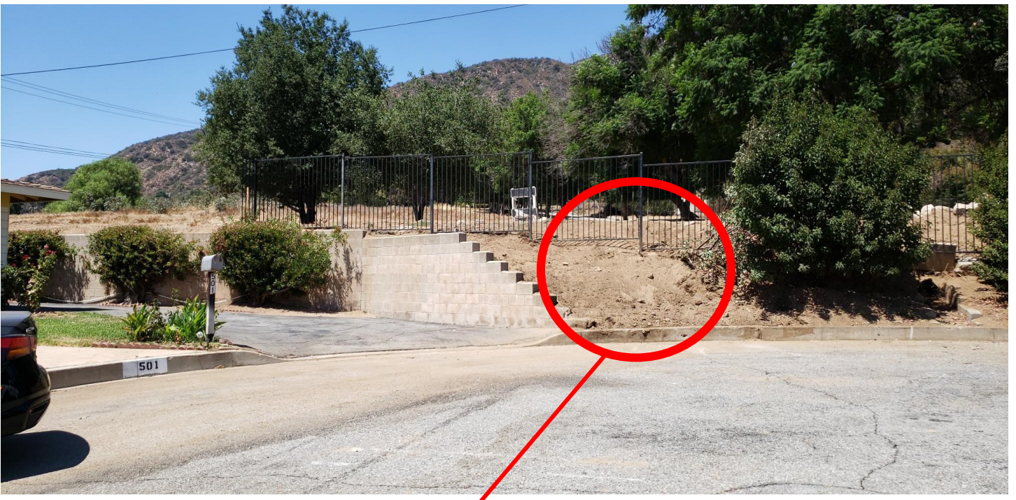
Water and Erosion Runoff at 501 Crestvale Drive. A boulder and brush were removed to repair; additional loose soil is now exposed. Flow pattern after the leak was repaired. 08/14/22.
