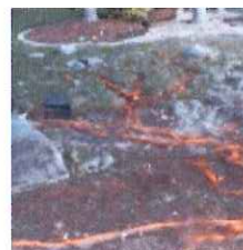
Root growth under the slab. Roots have been painted orange for
