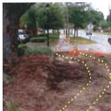
Once the roots have been exposed with an Air Spade, it is easier to determine the best location for the replacement sidewalk where the roots are smaller and less damaging to the sidewalk.
