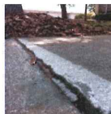
Shaving the lifted slab to even out the uneven edges is useful but only temporarily. Here a shaved slab is lifting again.
