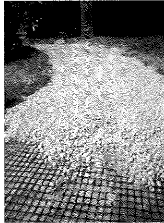
Installing geogrid mat over roots and then clean gravel provides a strong buffer against the lifting force of roots
